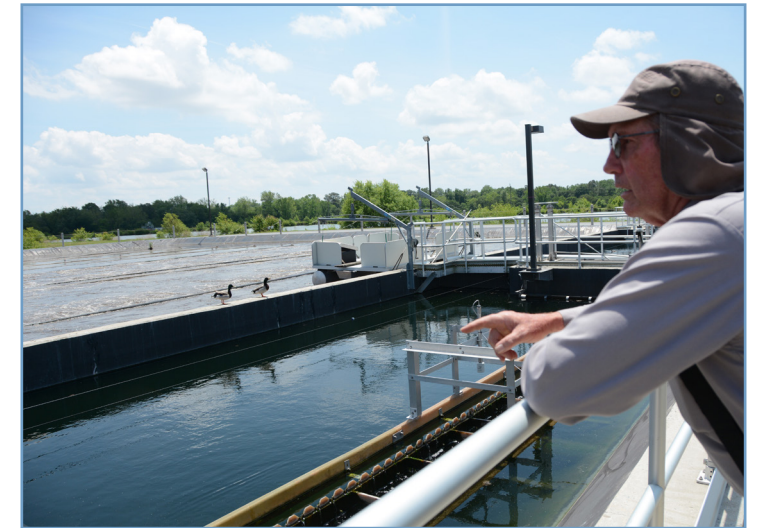
Laurel’s Wastewater Treatment Plant superintendent Mike Tipton monitors the plant’s sludge aeration process.
